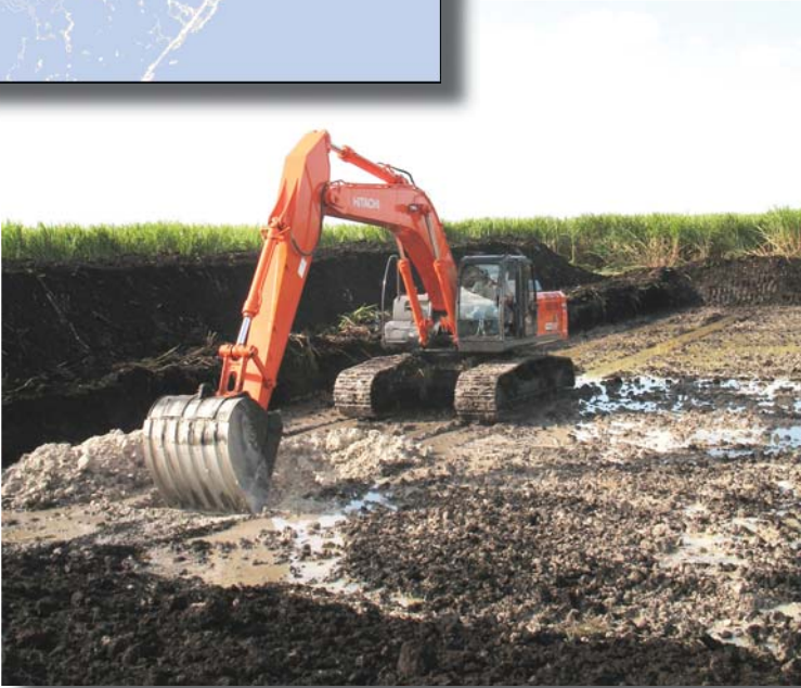
Figure 32: Excavation for a test mine on sugar cane land in western Palm Beach County (Source: LHC)
