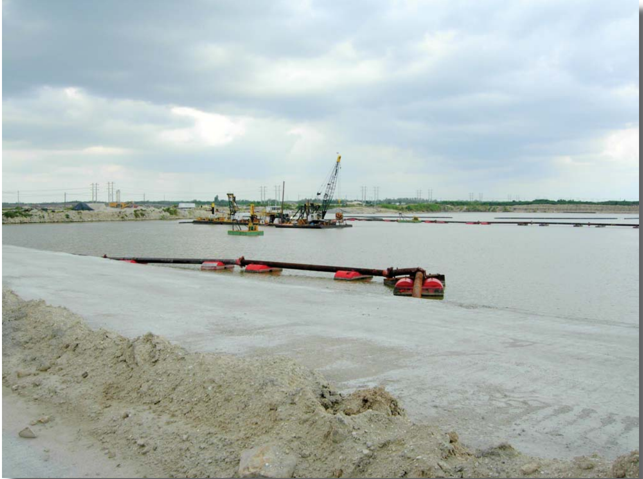
Figure 26: Creation of water storage reservoir at Palm Beach Aggregates Mine (Source: LHC)
